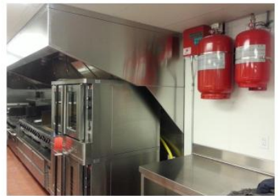
Kitchen Fire Suppression System
