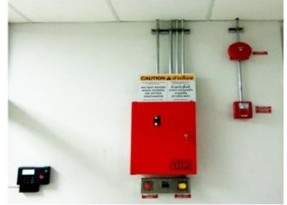
Fire Detection System
