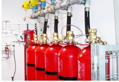
Clean Agent Fire Suppression System
