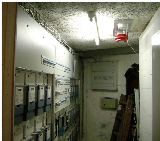
DSPA installed in the electric meter and fuse boxes in the basement of an apartment block.
